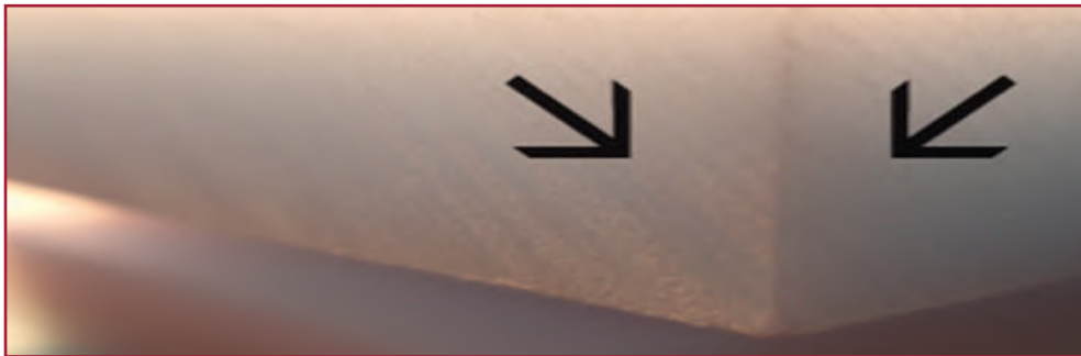
Fig.2 Shows marks from the cut with saw blade
